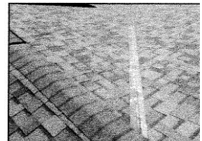
Section B - Deficiency #3 Deteriorated valley tin
